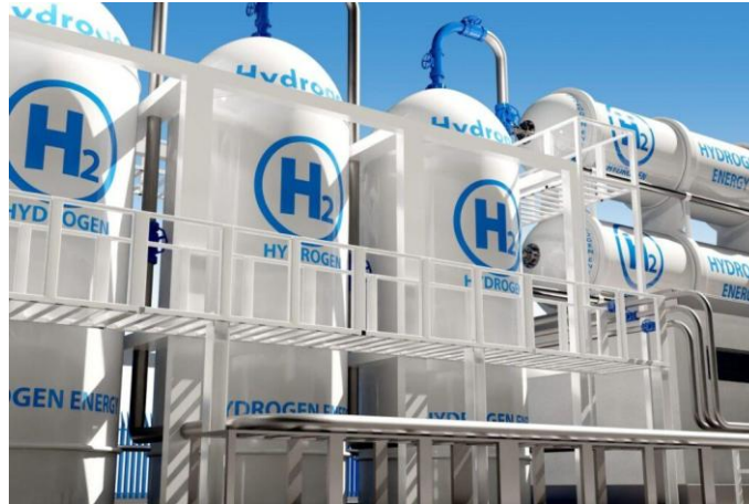
Figure 8: Example of hydrogen storage tanks 49 .
